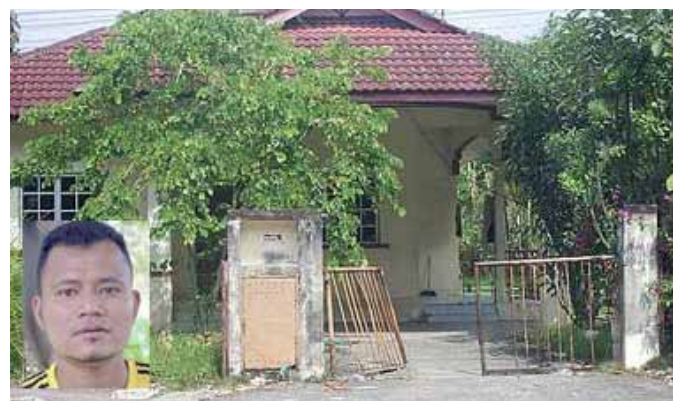
Not at home: One of the many dilapidated houses at the Orang Asli resettlement in Desa Temuan. Azman (inset) says the Orang Asli now reside in only 91 of the 147 houses. [From 'The Star Online']
